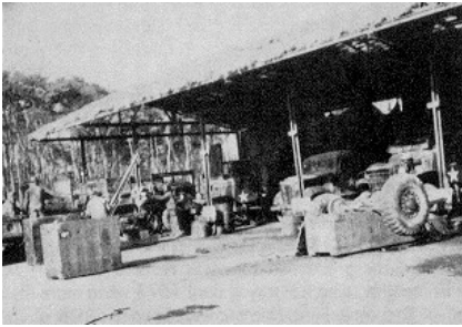
A bombed out railroad supplies the steel framework for this maintenance shop in Korea in early 1955.
